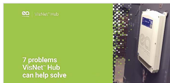
Figure 5. EA Technology 16kHz ‘VisNet’ Hub Installed at Port Talbot Sub-Station
